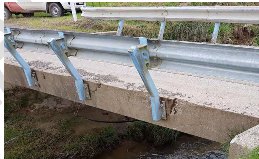
Figure 0-9 : Damaged side protection on Old Creamery Road bridge
