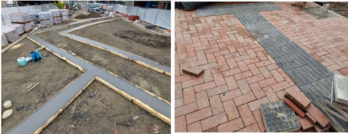
Progress images of the work on Church Street Town Centre Development (taken 17 July 2024).
