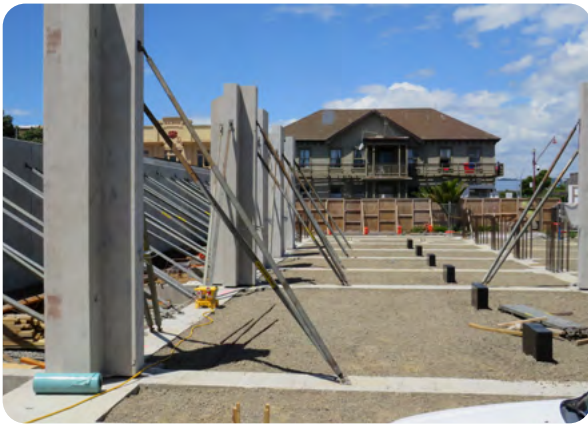
Photo below: Te Tāhuhu o Te Rangi is starting to take shape on the corner of King and Church Streets.
