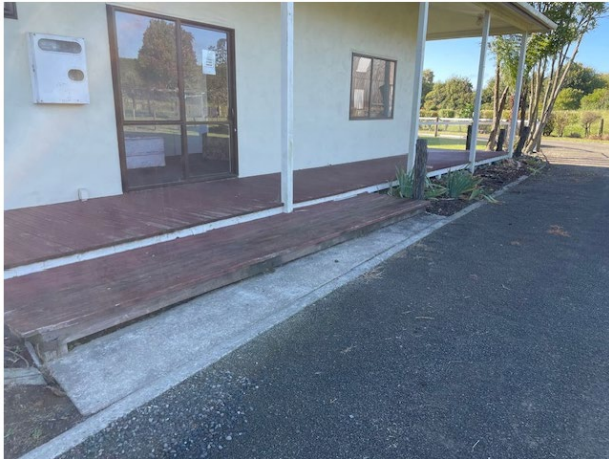
Figure 6: Photograph of ground and floor levels in the south-west corner of the building which is at the lowest level.
